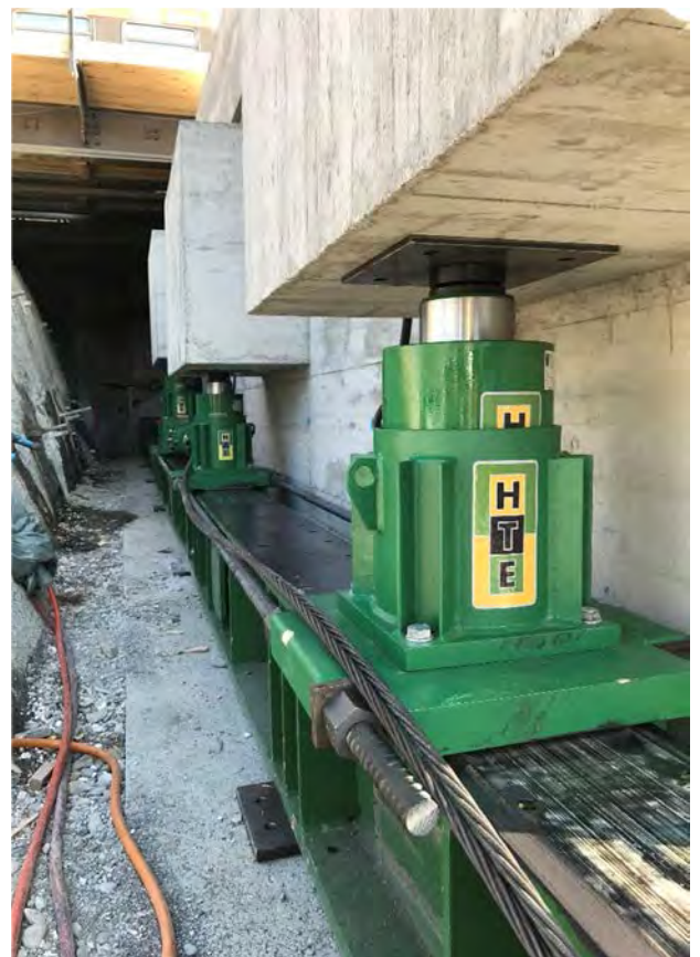
Sliding construction (Sliding beam, -shoe and hydraulic jack) with jacked up load during the sliding.
