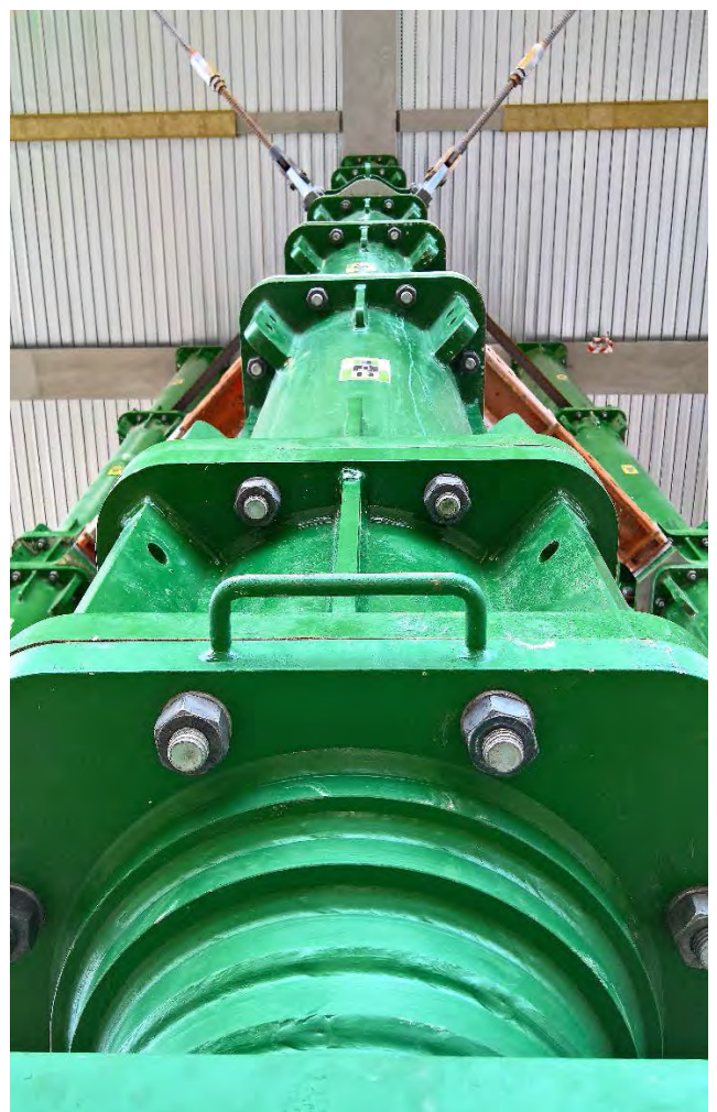
One of four columns of the total 19 lifting towers at final lifting height.
