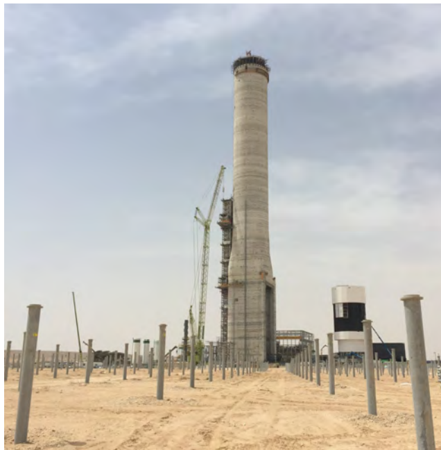
The concrete tower under construction using a slipform and the boiler assembly a few meters away.
